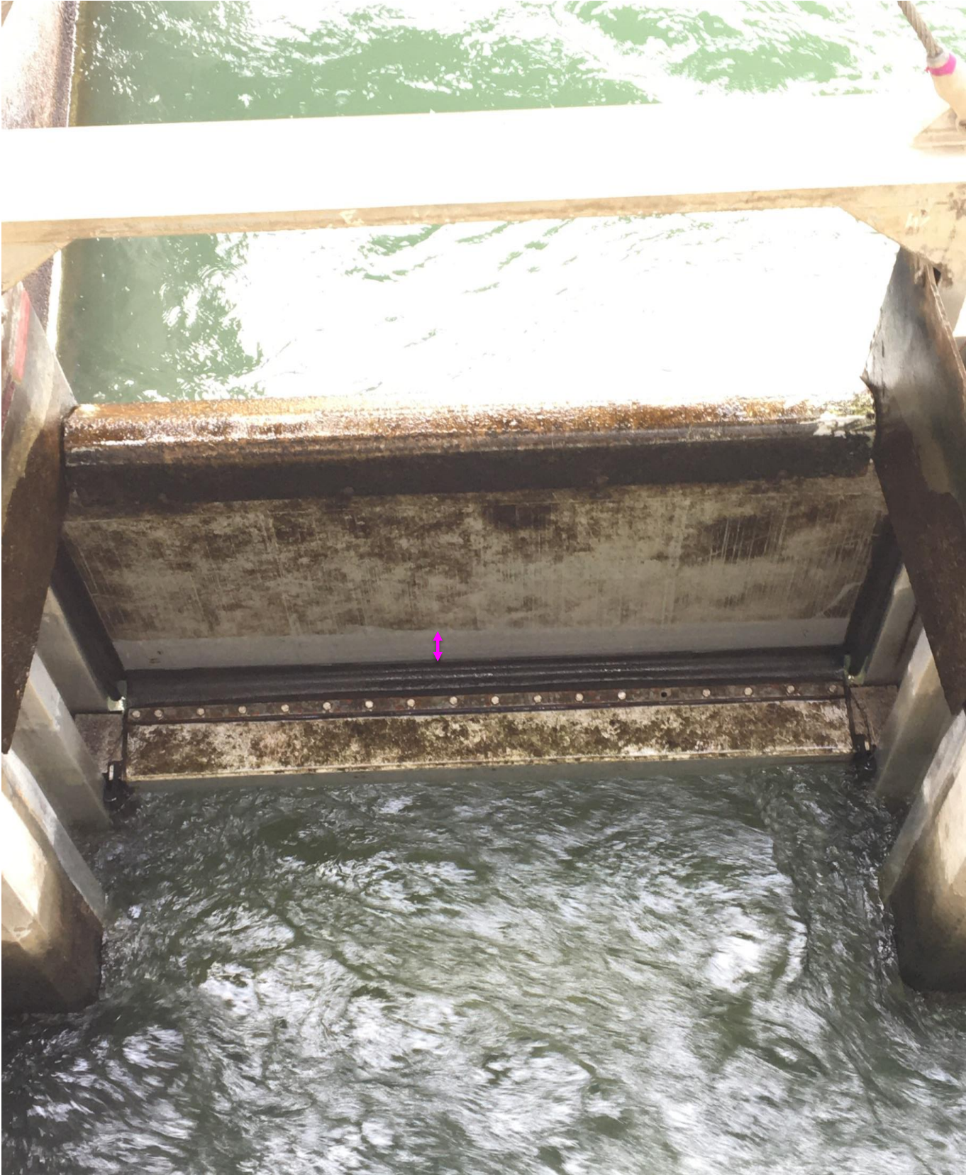
158 horizontal seal issue causing periodic binding.
